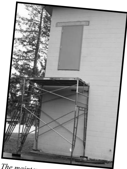
The maintenance department has added a new fire escape door to the outside wall of the choir rehearsal room. When the fire escape is attached, it will almost double the legal occupancy of the room
