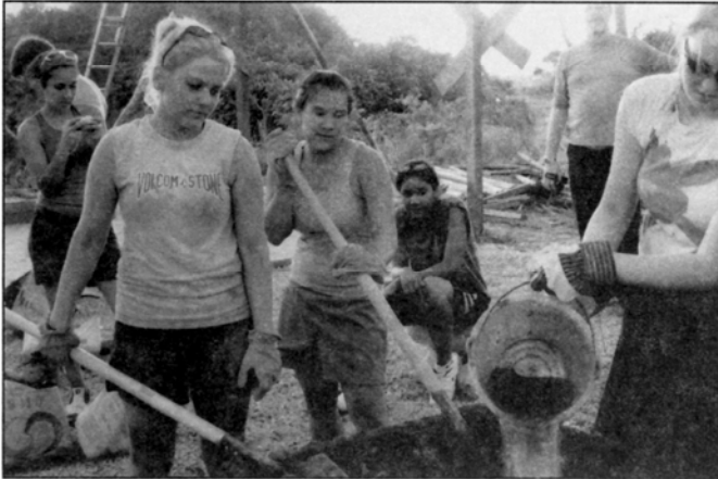
Jessica de Oro, Lacey Ringering, Katrina Yeo, Keity Hodgson and Cheria Hunter work at the church building site in Borneo
